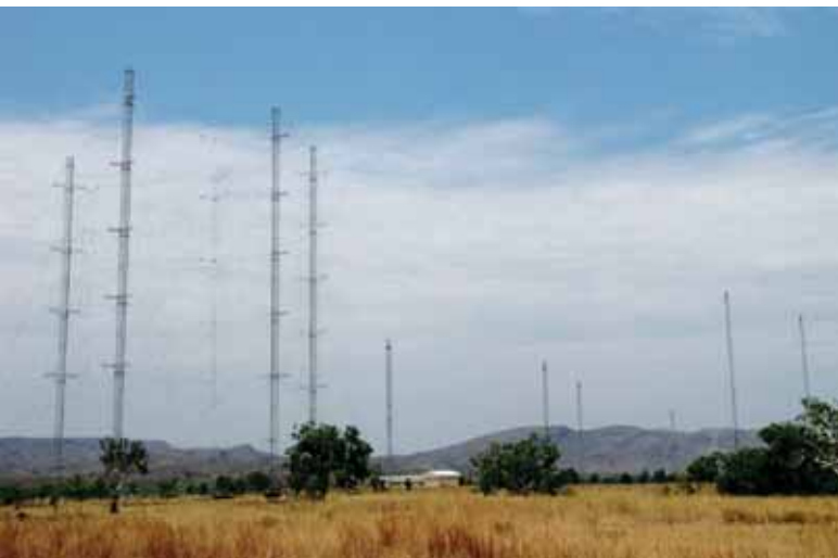
Kununurra Antenna Farm as at 27 Oct 2011: Four towers on left have aeriels erected on them, as do two towers on extreme right. Others will be erected as time permits.
